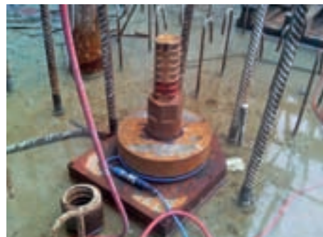
Anchor with Sensor Unit
