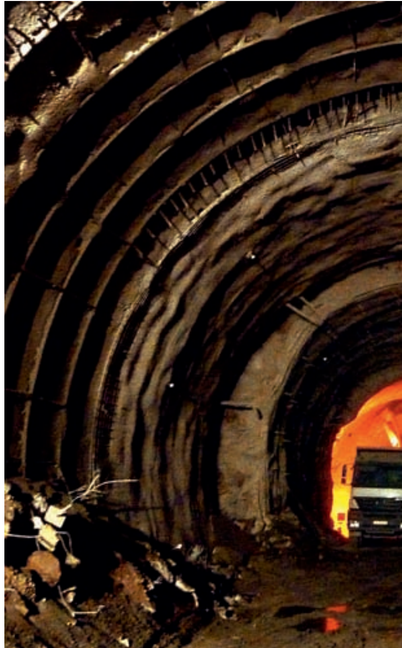
Support of Tunnel Lining using IBO - Self-Drilling Anchors and PANTEX Lattice Girders
