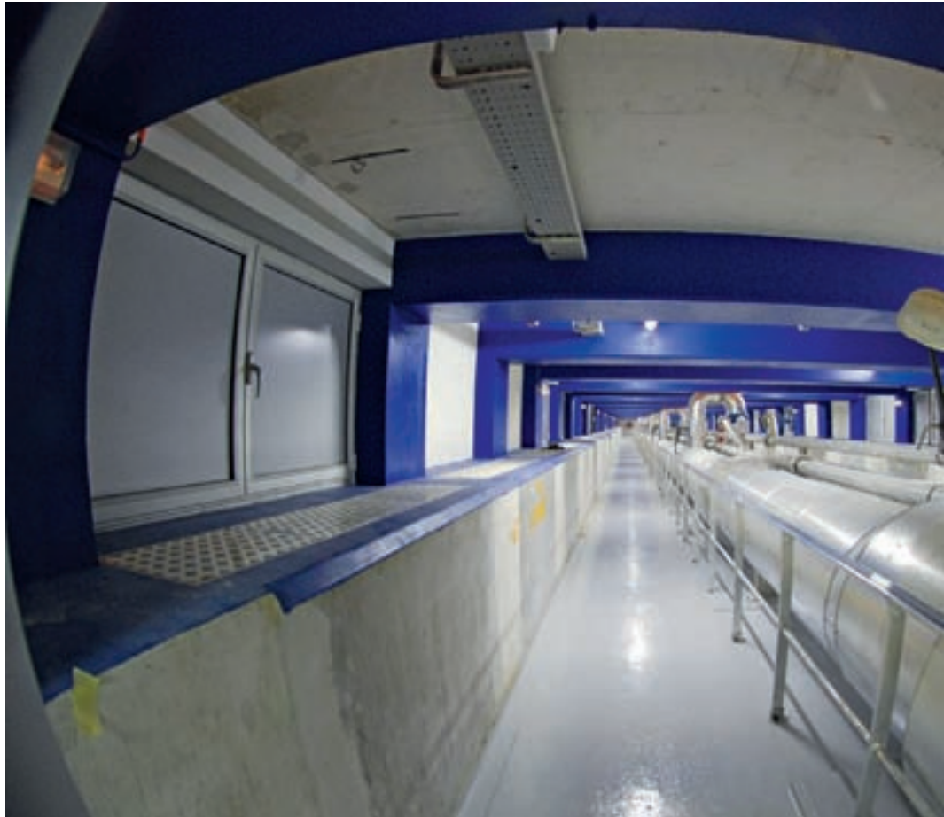
Sealed surfaces in subterranean sewage plant
