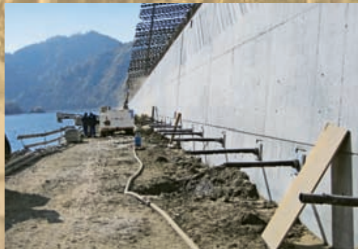
Partially stressed anchor
