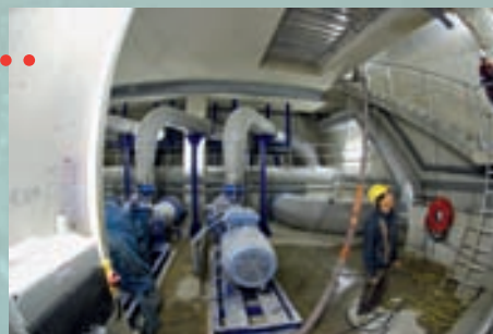
View into pump room
