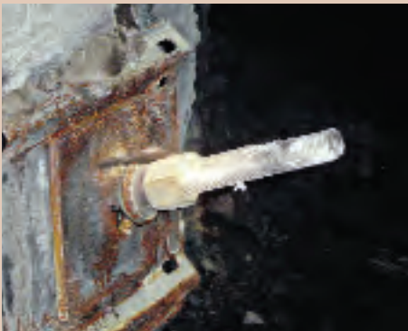
That's how far the old rib bolts at Beltana mine protruded
