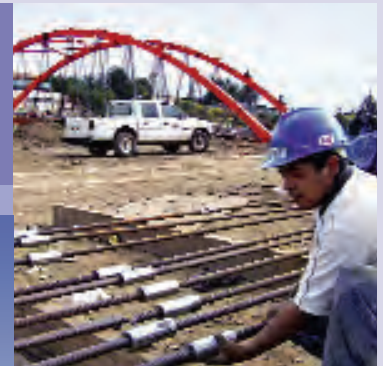
Preparation of DYWIDAG Bar Tendons at the Alcides Carrión bridge in Huánuco, Peru
