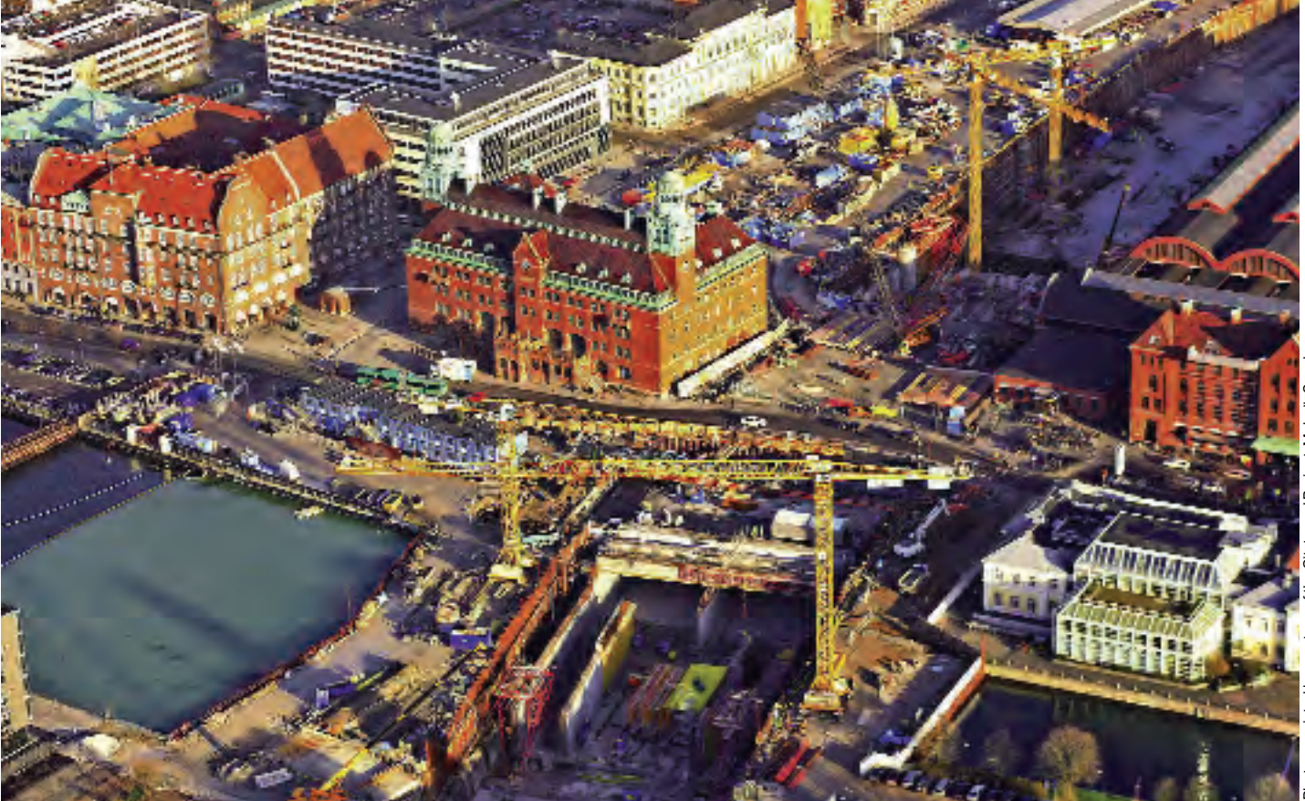
Photos reprinted by courtesy of the Citytunnel Project, Malmö, Sweden, of NCC Construction Sverige AB, Malmö, Sweden, and of Brückner Grundbau GmbH, Essen, Germany
